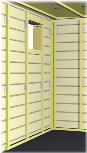
1. Fasten battens to the log wall with sliding angle brackets as shown on T18.
